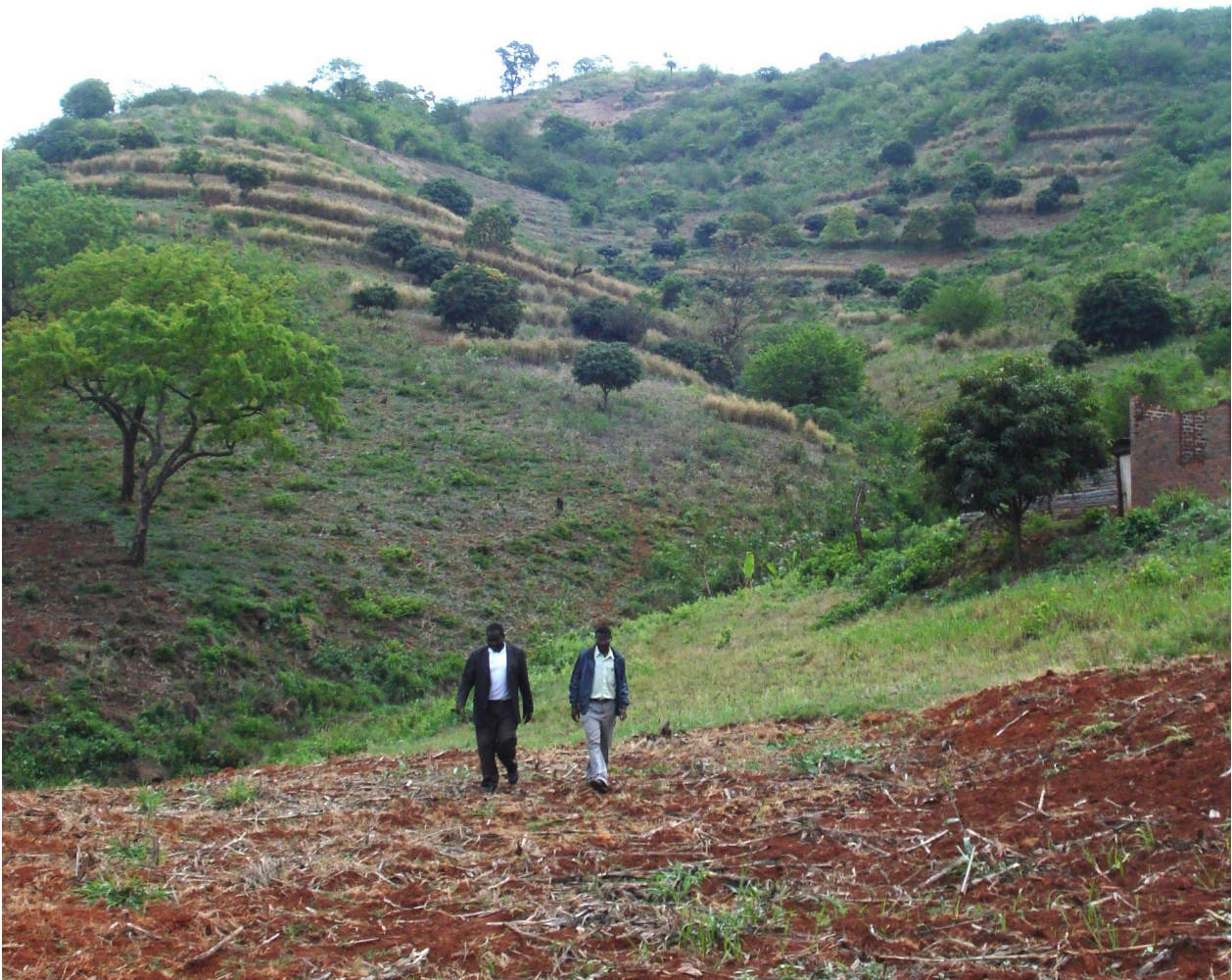
Vetiver grass bunds and gabions constructed on steep slopes by the Landcare group at Khumbe , Limpopo Region in South Africa.
